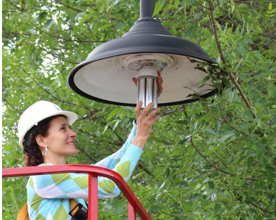
Example of an LED streetlight (City of Woonsocket)
