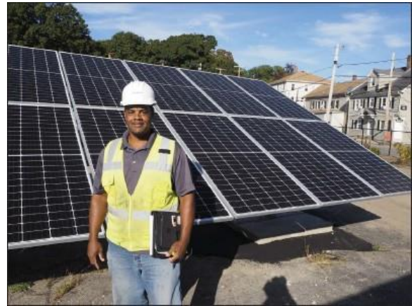
Solar array at former Alice Mill site, Fairmount Street, Woonsocket (The Call)
